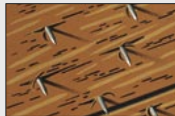
Nail holes and joints in your roof deck provide the channels for water to seep through.
